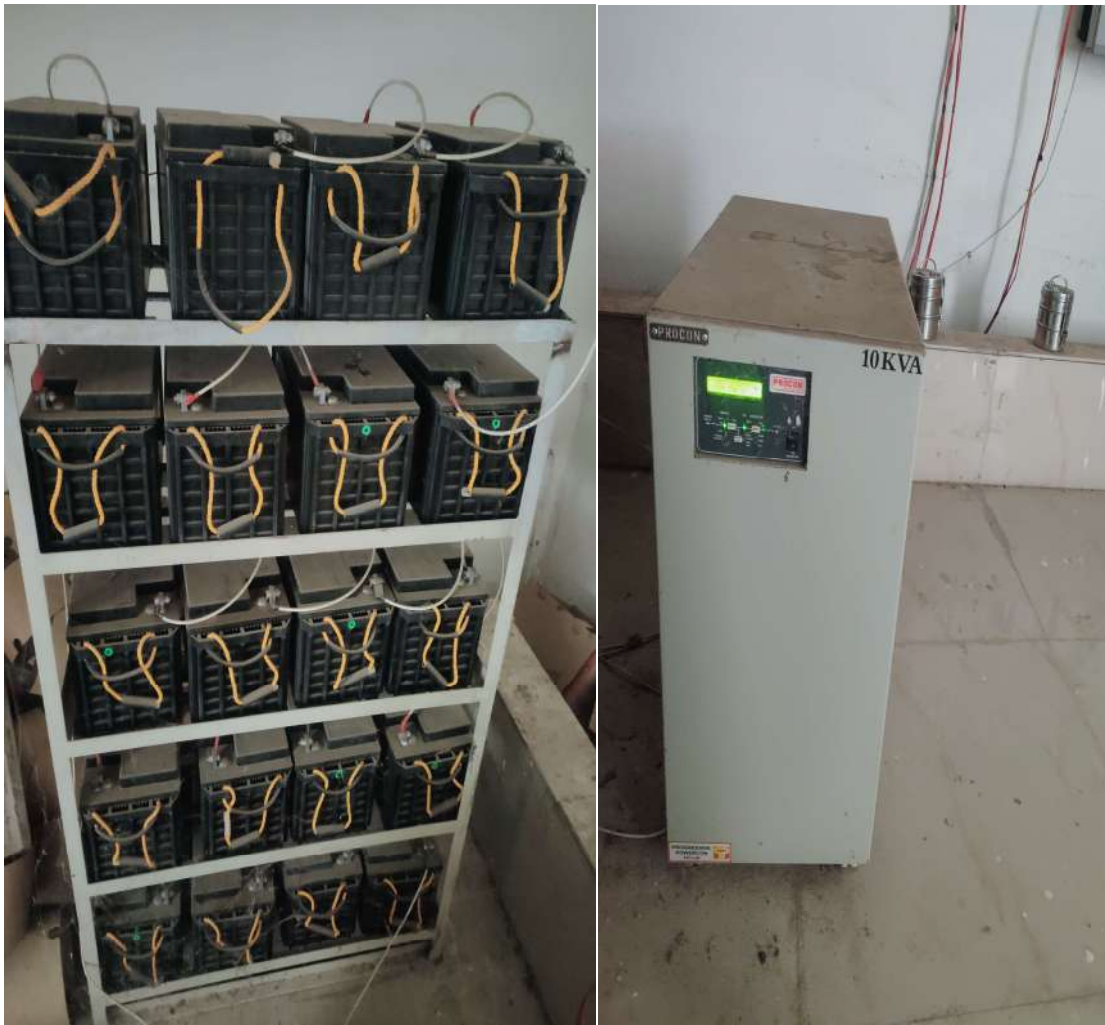
10 KVA UPS with batteries for uninterrupted power supply
